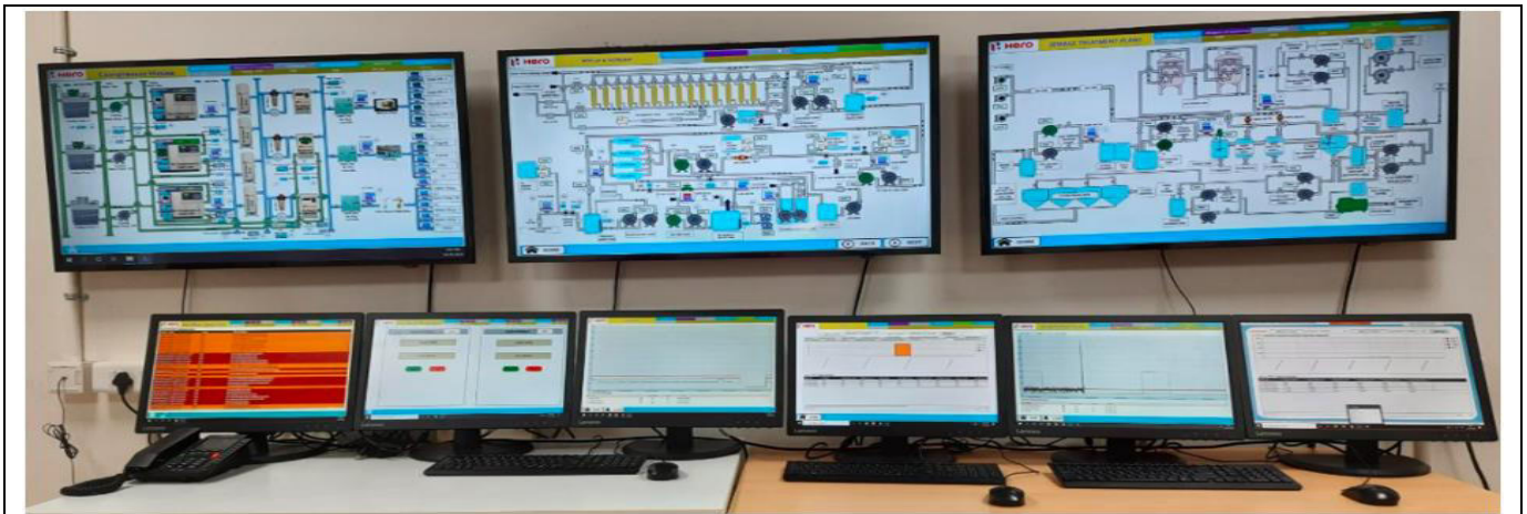
Utility Monitoring & Controlling Systems
